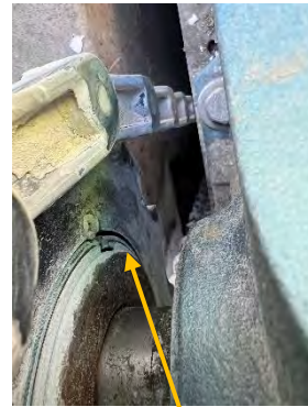
Failed Shear Pin Assembly
