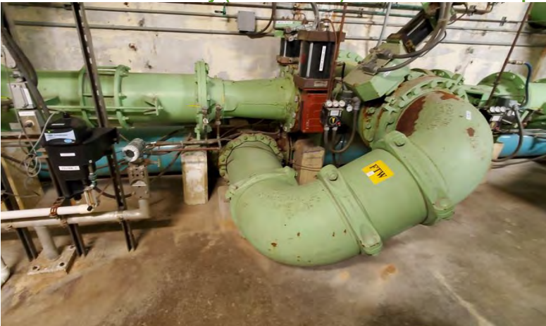
Photo 13: Filter Gallery (Filters 1 - 10) – Filter Effluent Flow Metering & Control Valves
