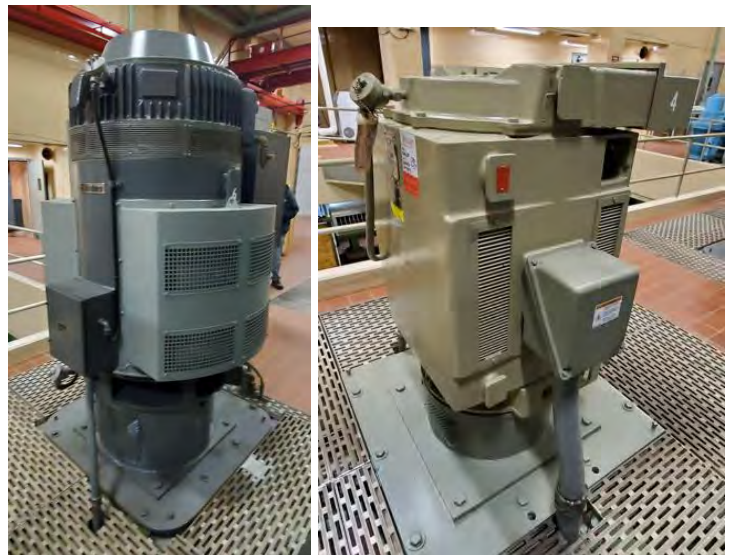
Photo 15: High Service Pump 3 & 4 Motors
