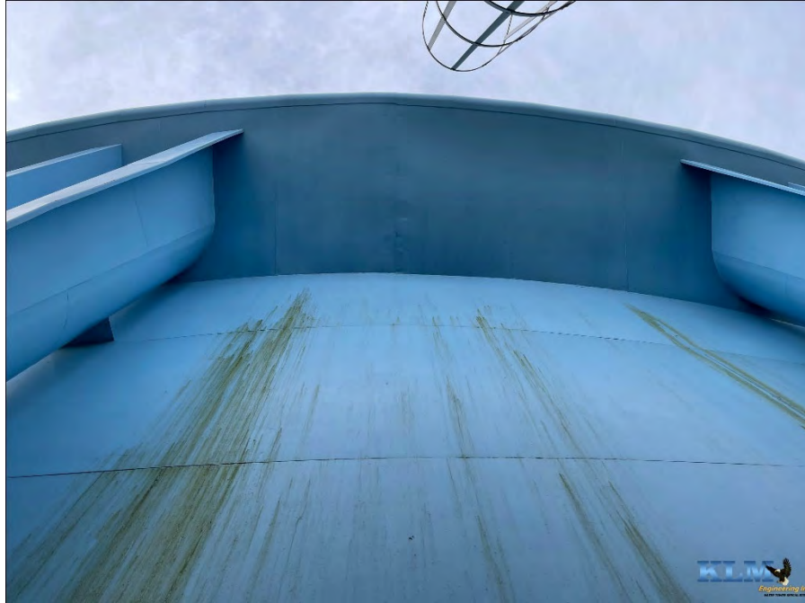
Photo No. 29 Shell exterior conditions with dirt accumulation visible
