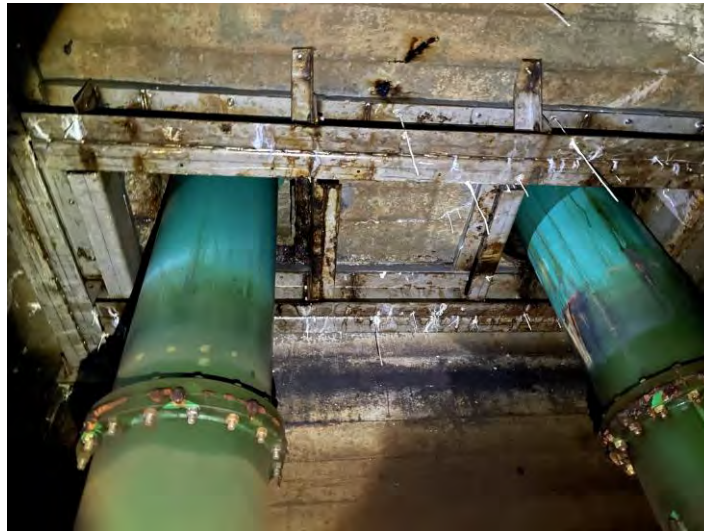
Figure 13 Rust at retrofit pipe opening framing
