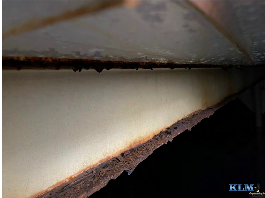
Photo No. 7 Condition of rafter
