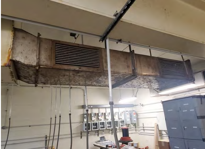
Photo 20: Lime Slaker Room – HVAC Corrosion
