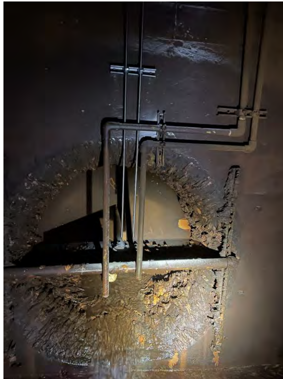
Figure 19 Effluent piping tuberculation
