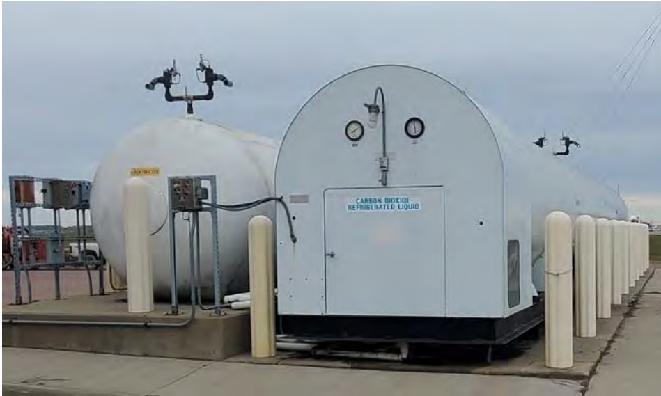
FIGURE 21: CARBON DIOXIDE STORAGE TANKS
