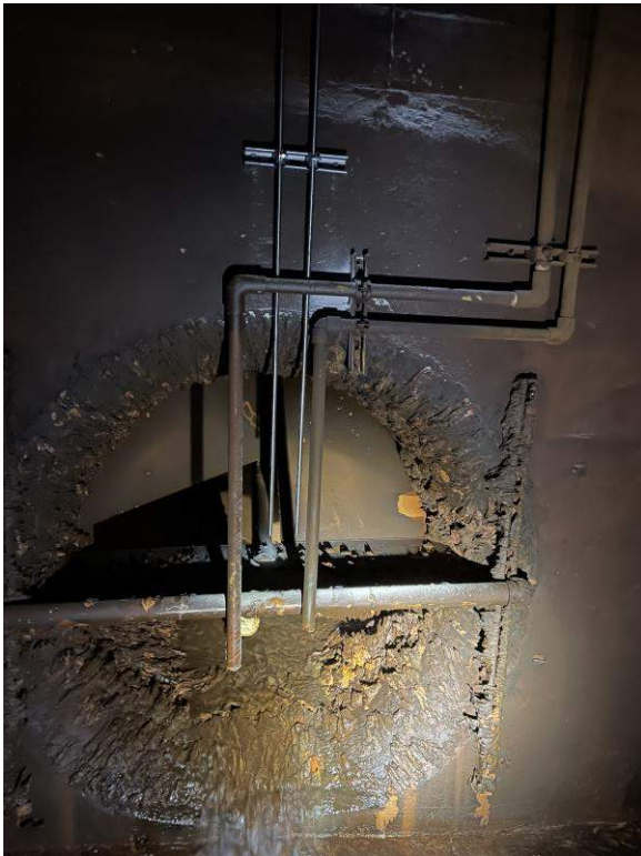
Figure 19 Effluent piping tuberculation
