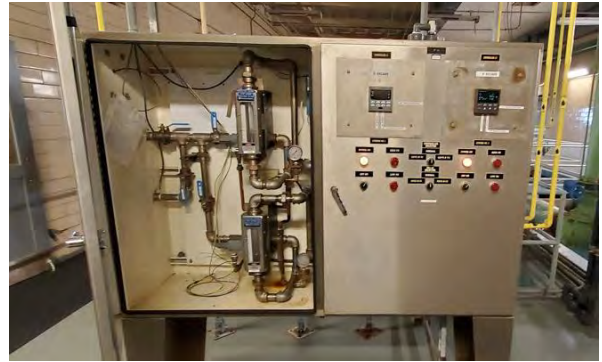
Photo 7: CO 2 Feeder Equipment
