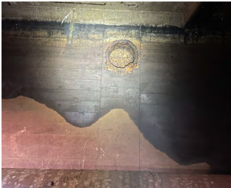
Figure 14 Example of an abandoned pipe
