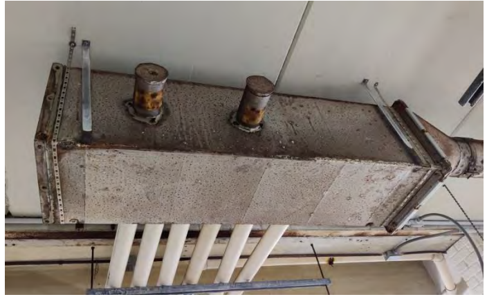
Photo 21: Lime Slaker Room - HVAC Corrosion
