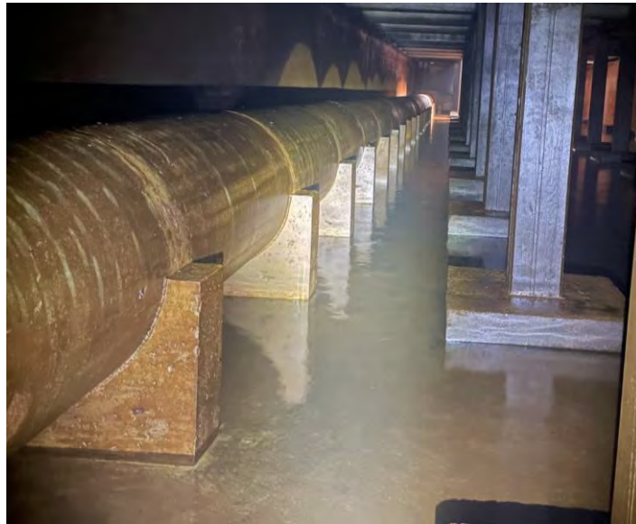
Figure 16 Influent piping concrete supports
