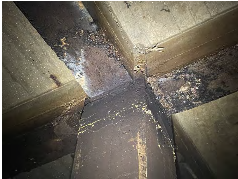
Figure 8 Unconsolidated concrete and exposed aggregate
