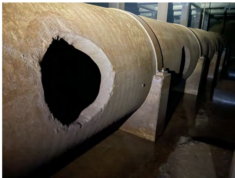
Figure 17 Influent piping openings
