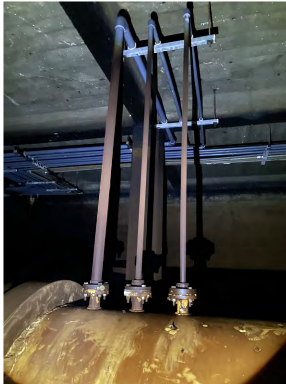
Figure 26 Clearwell influent chemical feed
