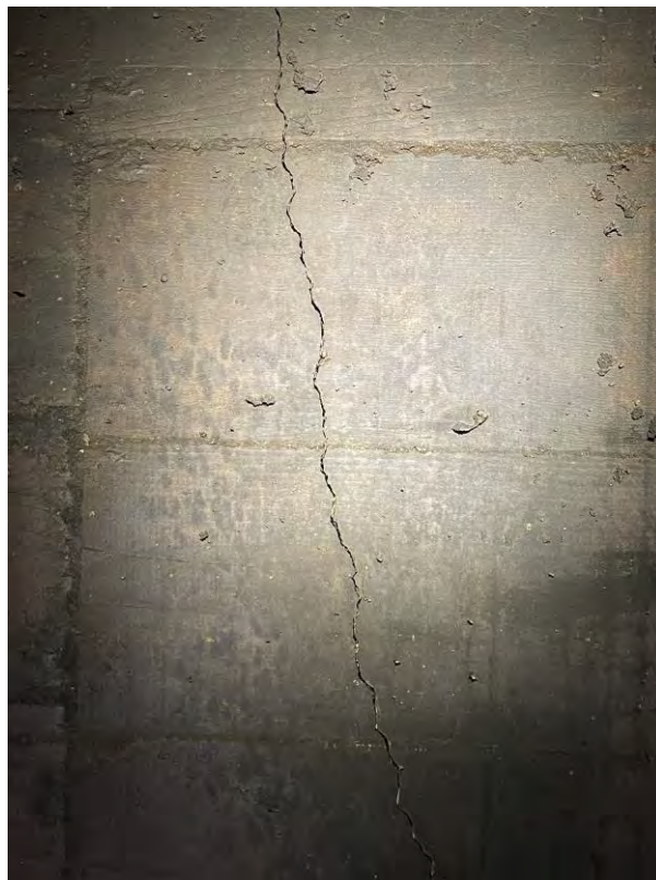
Figure 7 Vertical crack in concrete baffle wall
