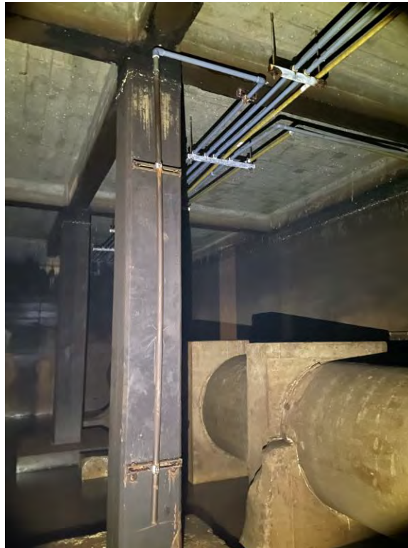
Figure 29 Clearwell effluent sample piping
