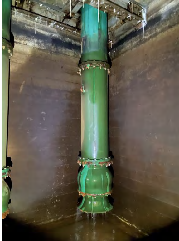
Figure 21 Backwash supply pumps
