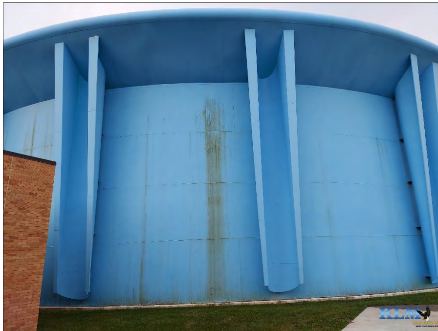
Photo No. 30 Shell exterior conditions with dirt accumulation visible
