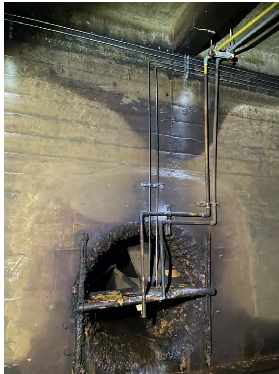
Figure 27 Clearwell effluent chemical feed
