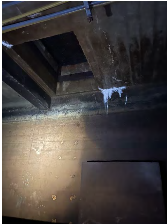
Figure 4 Mineral intrusion at crack in roof slab
