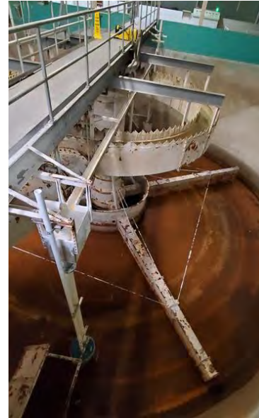
Photo 3: Solids Contact Basin Sludge Scrapers
