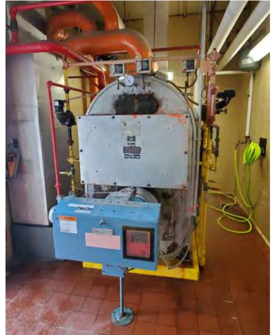
Photo 28: Facility Boiler (High Service Pump Area)
