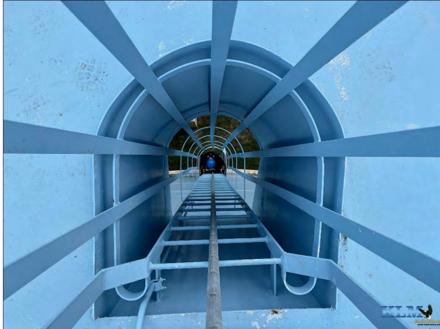
Photo No. 25 Exterior roof ladder access and cage conditions
