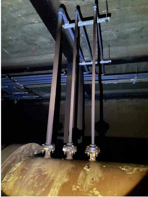
Figure 26 Clearwell influent chemical feed
