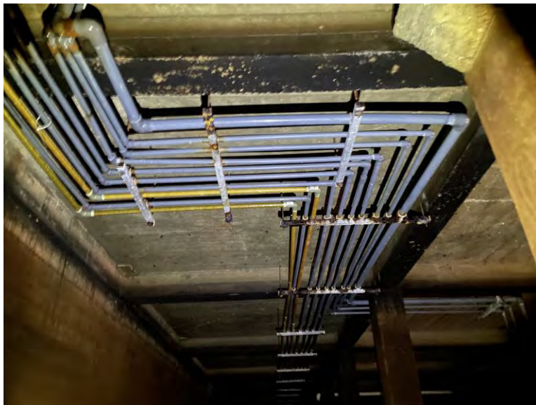
Figure 25 Chemical piping (within clearwell)
