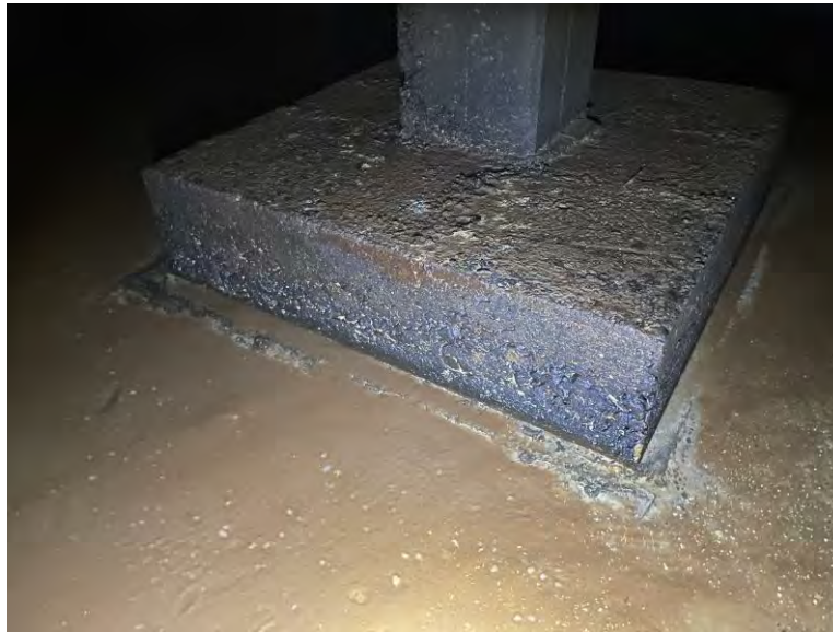
Figure 10 Spalling at concrete column pedestal
