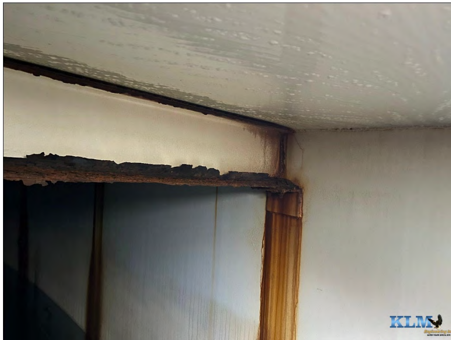
Photo No. 8 Typical condition of rafter and support angle
