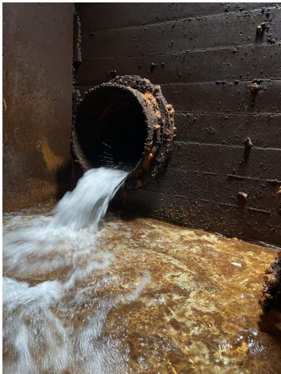
Figure 20 Clearwell effluent pipe (valve closure issue)
