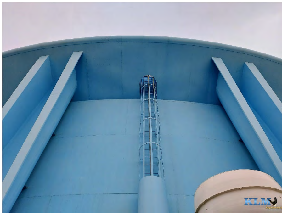
Photo No. 26 Exterior ladder and cage conditions
