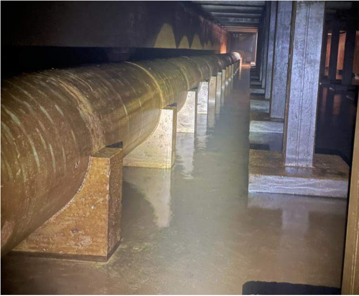
Figure 16 Influent piping concrete supports
