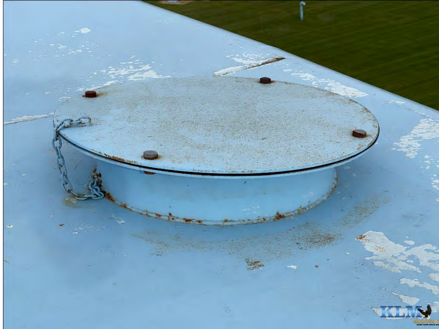
Photo No. 19 Ventilation manway
