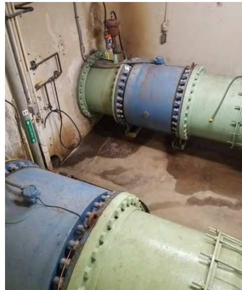
Photo 2: INFLUENT FLOW METERS (36-INCH DIAMETER)
