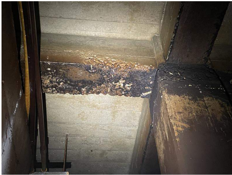
Figure 9 Unconsolidated concrete at beam
