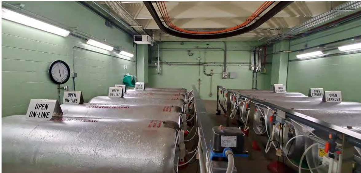
FIGURE 22: CHLORINE STORAGE ROOM
