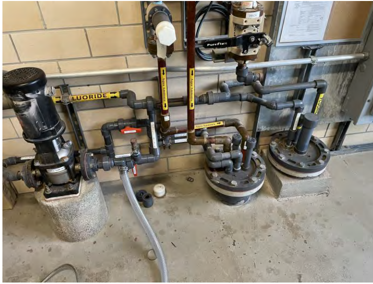
Figure 24 Chemical piping (above clearwell)
