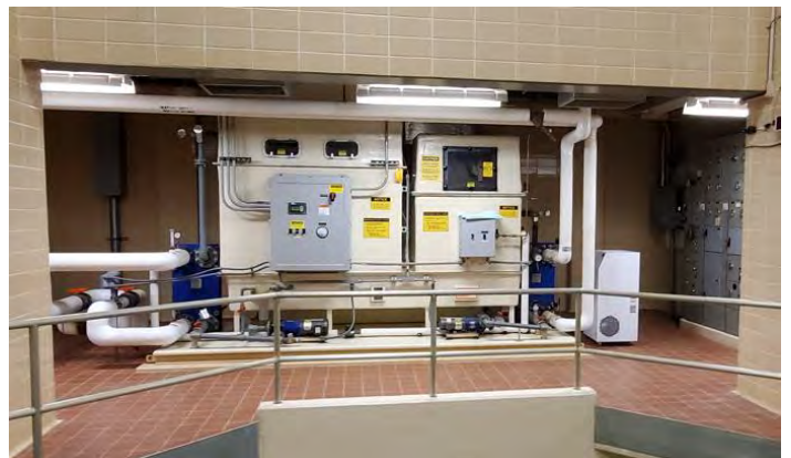
Photo 16: Kathabar Dehumidification System
