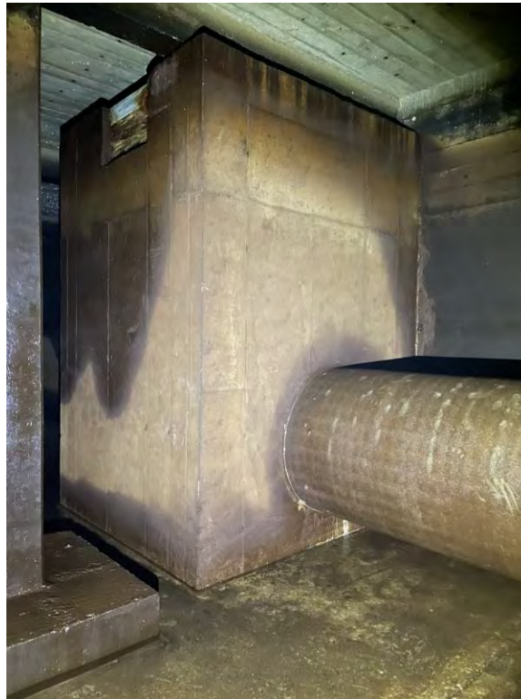
Figure 15 Influent box and influent piping
