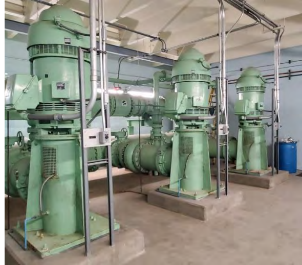
Photo 17: Transfer Pumps (North Reservoir)
