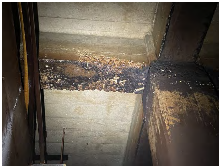
Figure 9 Unconsolidated concrete at beam
