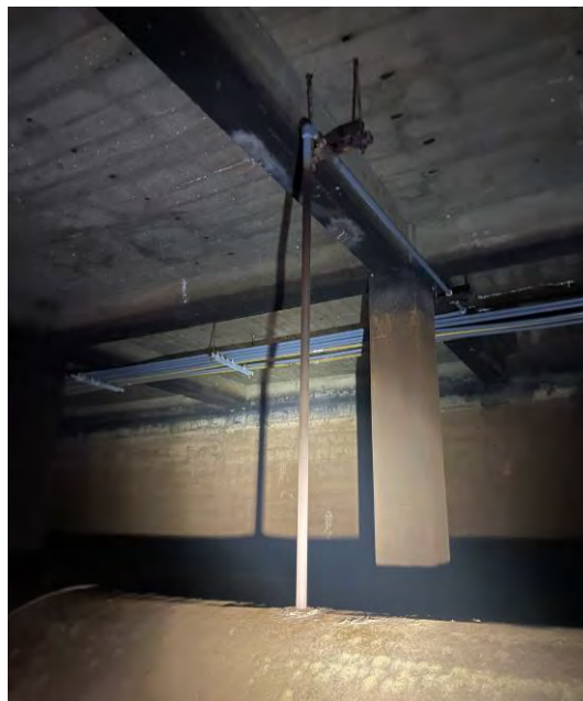
Figure 28 Clearwell influent sample piping
