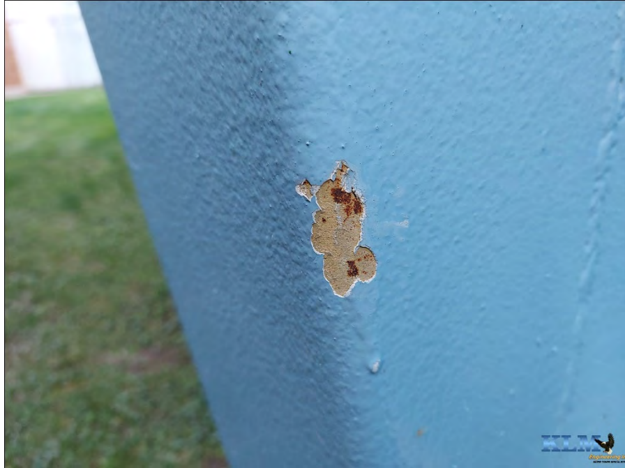
Photo No. 31 Layers of exterior coating shown at damage location
