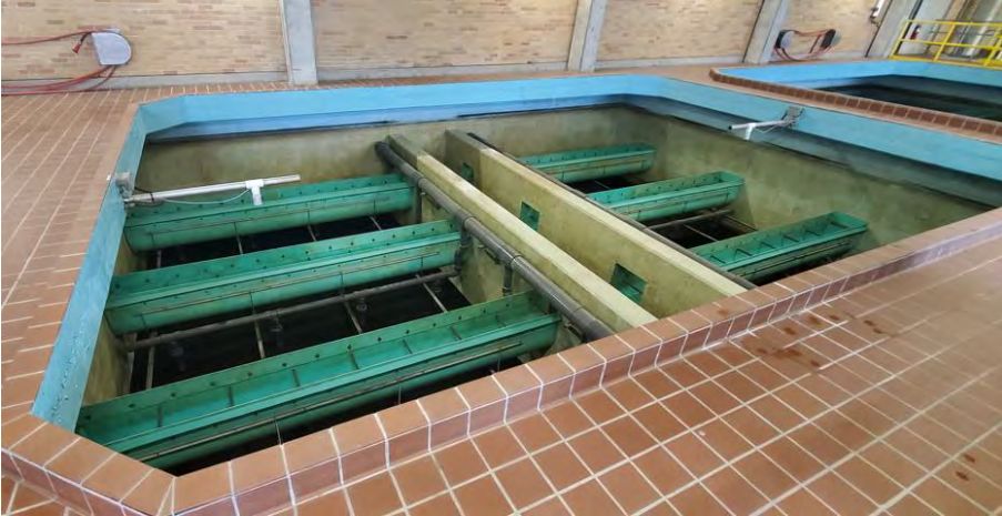
Photo 11: Filter 12 Backwash Troughs
