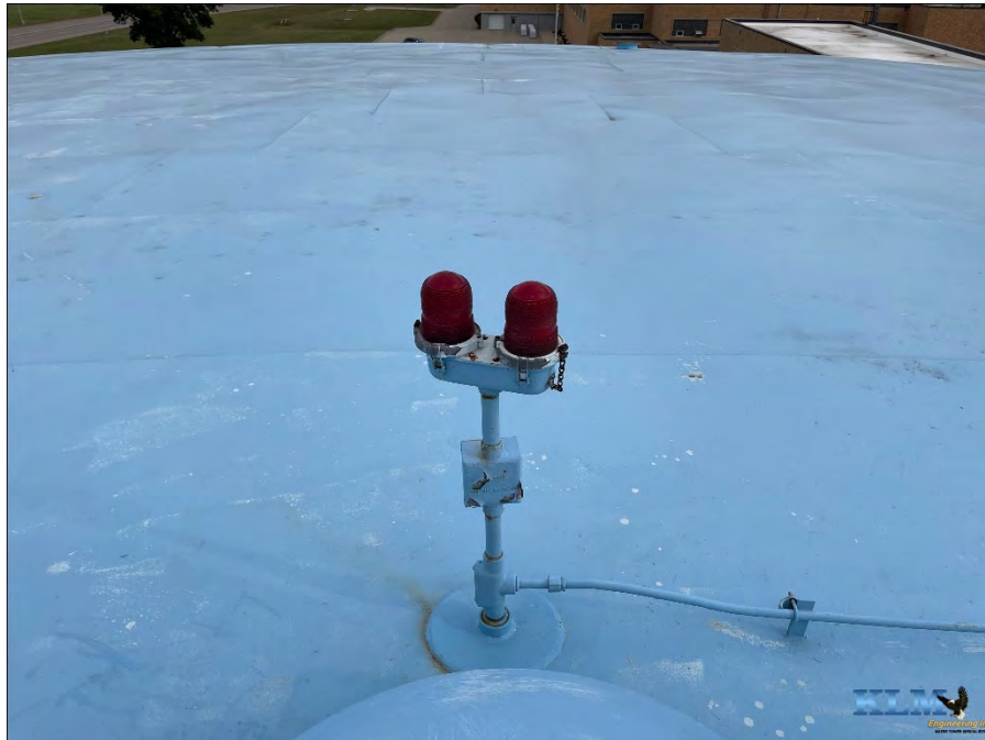
Photo No. 20 Aviation lights on roof
