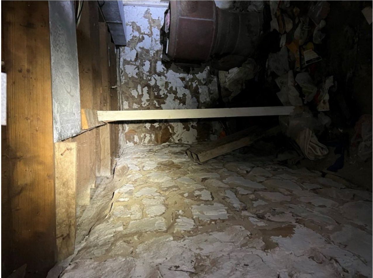
1025 S. Dakota Avenue Grout deterioration observed in west stone foundation wall
