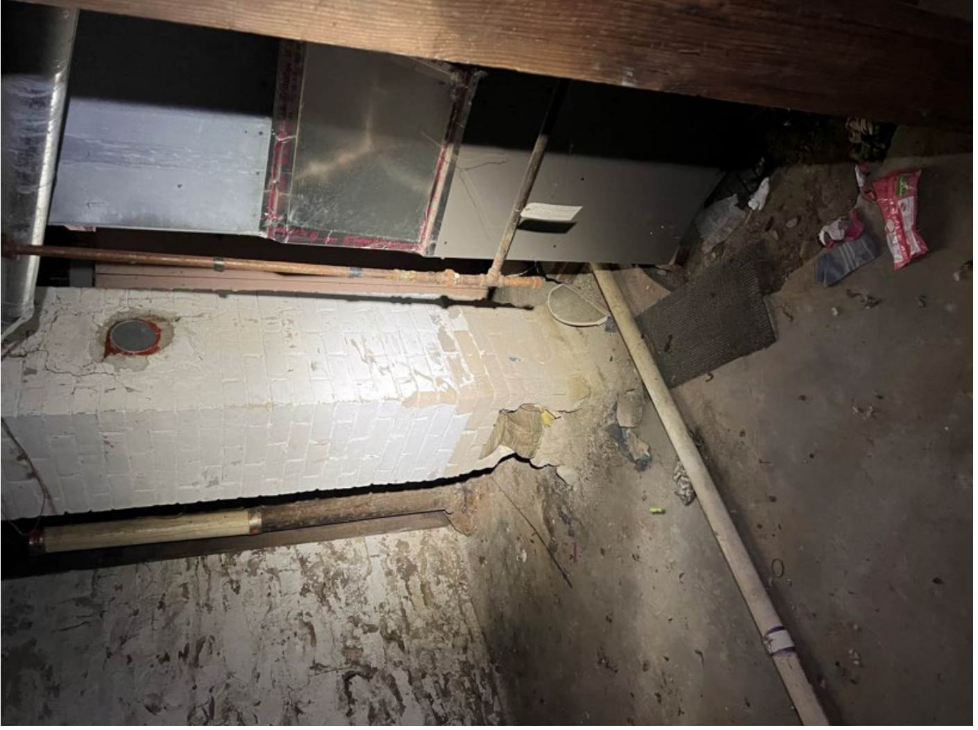
1005 S. Dakota Avenue (right) Deterioration at base of chimney structure
