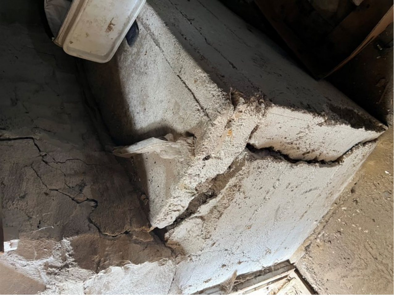
1025 S. Dakota Avenue Foundation wall cracking in west foundation wall
