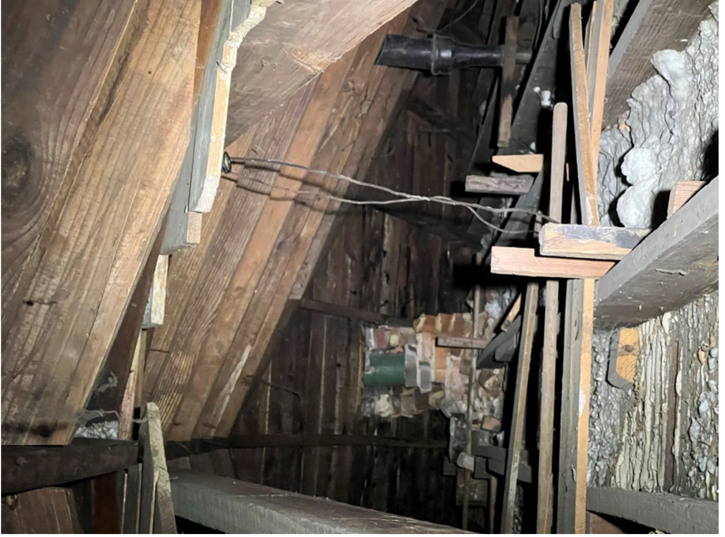
414 West 19 th Street Chimney structure observed to have partially collapsed within roof structure
