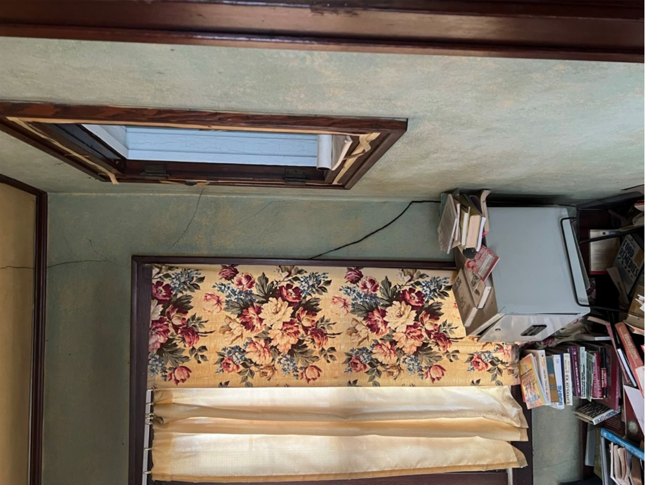
414 West 19 th Street Significant exterior wall cracking was observed at east and west wall
